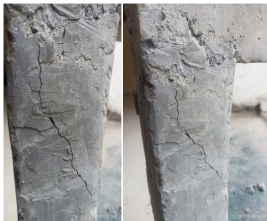
Fig no –5.0 (A) showing formation of crack
