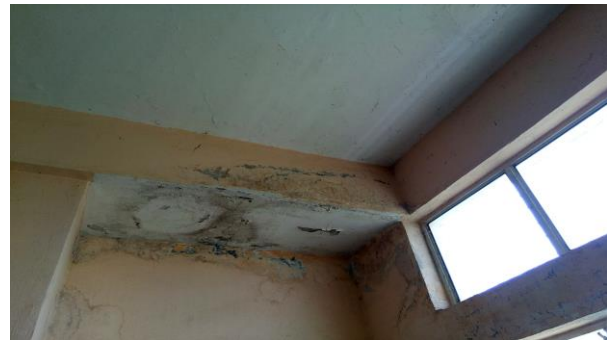
Fig.2.1.5 Defect occurred due to Dampness
