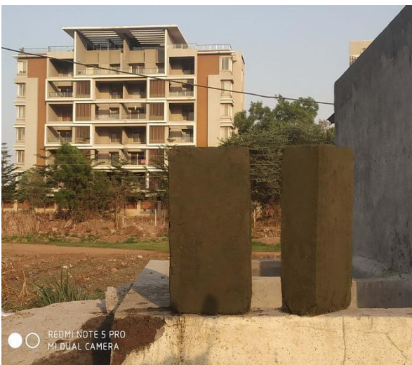
Fig No. 9 (Even surface obtained after plastering the columns casted using embossed plate formwork)
